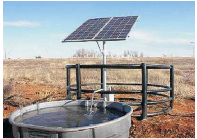
Solar Panels Provide Power In Remote Areas
